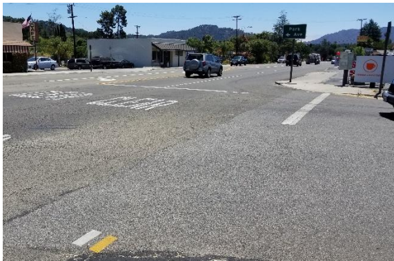
Figure 19: Incomplete limit lines and missing pedestrian crosswalk
