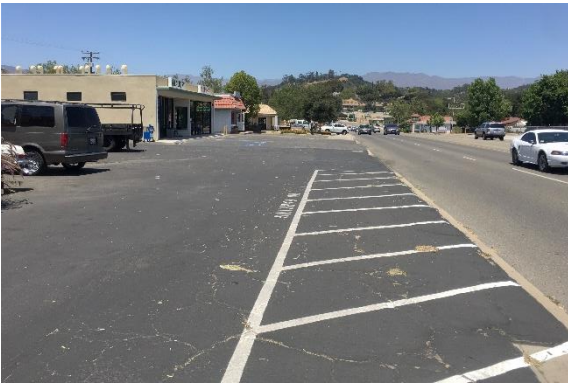
Figure 8: Options for pedestrians in study area extremely limited, such that they are forced to use the asphalt of a parking lot as a walkway.
